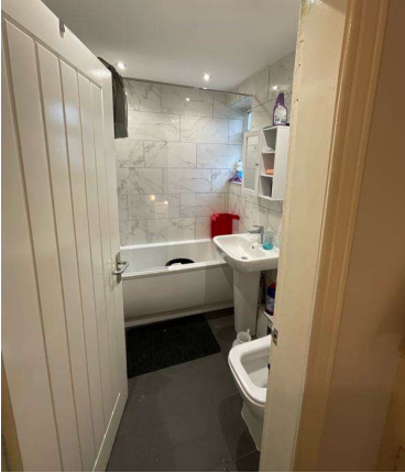
07-10-2023 13:36 / Bathroom Walls / Ceilings / 363iqa8ip
